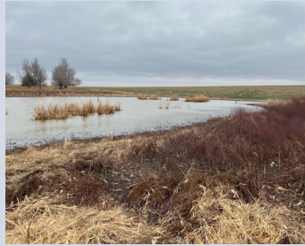
A sink hole developed at the site of an unplugged disposal well at the French site in Stafford County. The site is classified as moderate-high immediacy.
